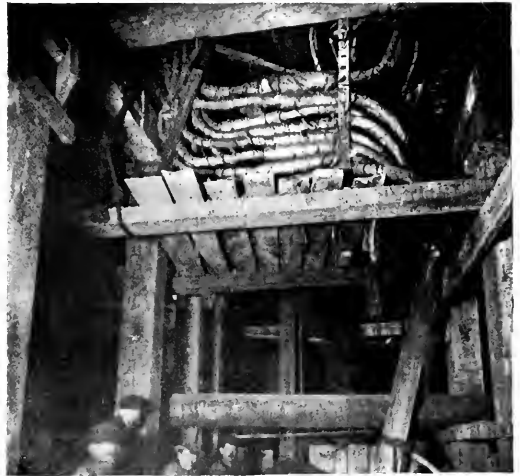
FIG. 1.—CABLES AT SCENE OF THE FIRE.
